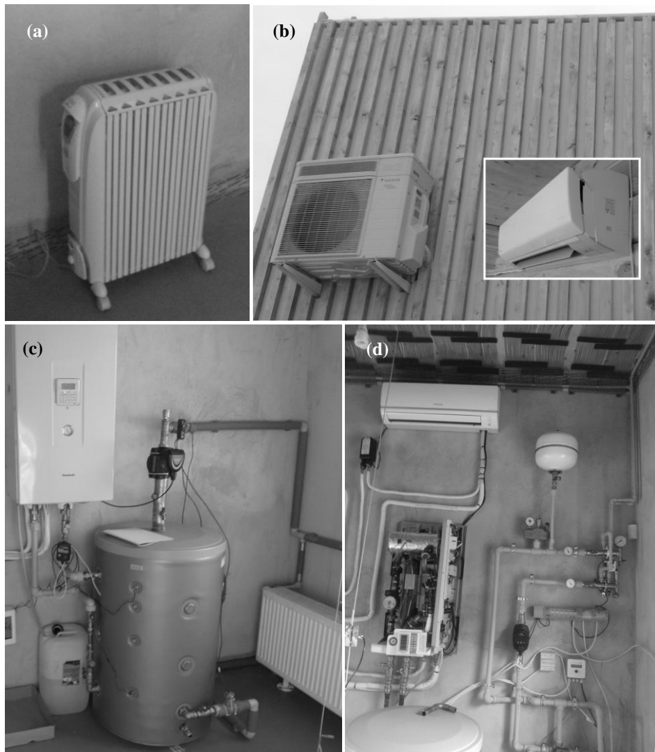
Fig. 2. Different heating systems investigated: (a) electric heater, (b) air-air heat pump, (c) air-water heat pump with convectors, (d) air-water heat pump with capillary mats placed on the ceiling.
